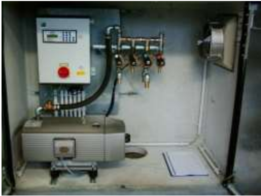
Figure 1: Inside of two-door concrete cabinet
