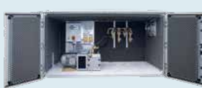
Concrete external cabinet
