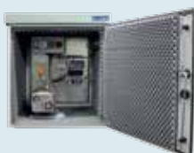
L metal external cabinet
